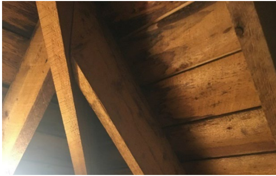
Rafter and boards of original roof seen from attic in original building.
