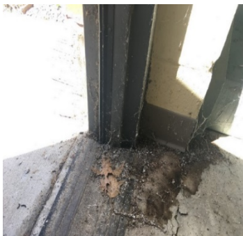
Threshold at rear egress door with damaged concrete slab.
