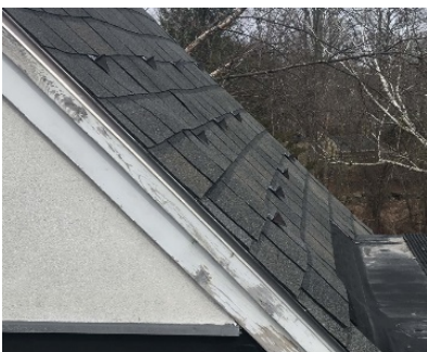
Rippled asphalt shingles on entrance gables.
