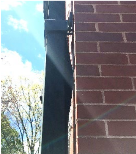
Open seam at back of downspout.
