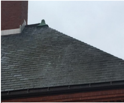
Lichen growing on north side of slate roof.
