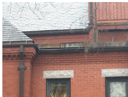
Damaged gutter and flashing on west elevation of flat roof.
