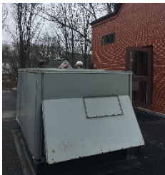
Rooftop Ventilation Unit
