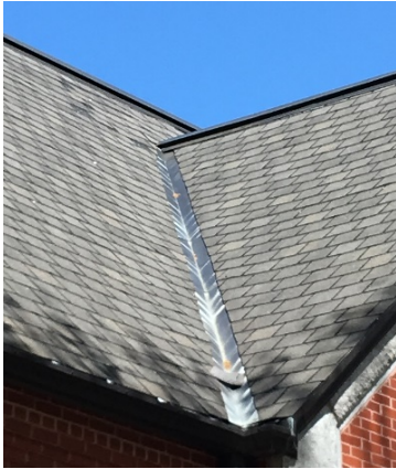
Asphalt shingles rippling and falling in roof addition.
