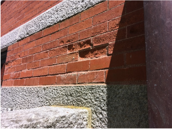
Figure 14 - Spalling bricks SW corner of original building.
