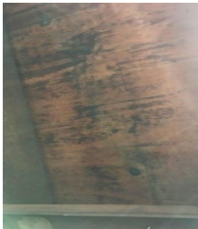
Mildew growing on plywood of roof deck over gabled entrance.
