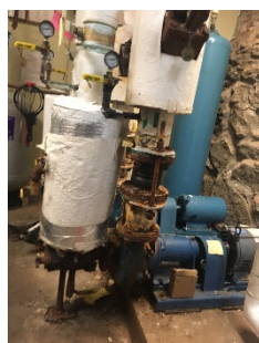
Part of HVAC system that is corroded.
